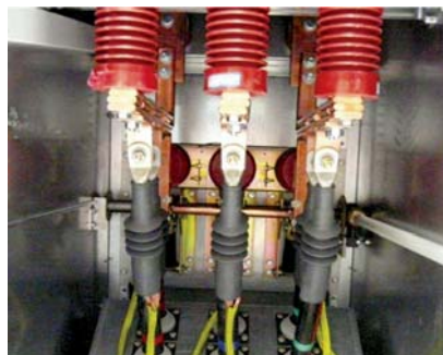
Connected power cable to the feeder busbar
