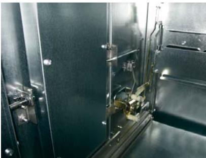
Interlock for circuit breaker compartment door
